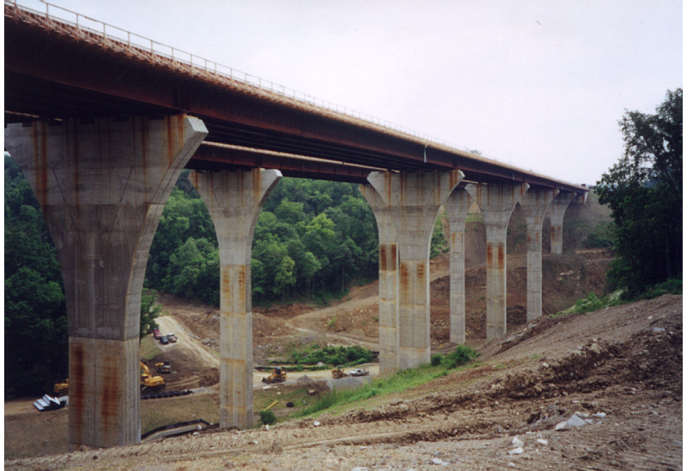
Dual bridge structures at Section 52-E of the Mon Fayette Expressway under construction.
