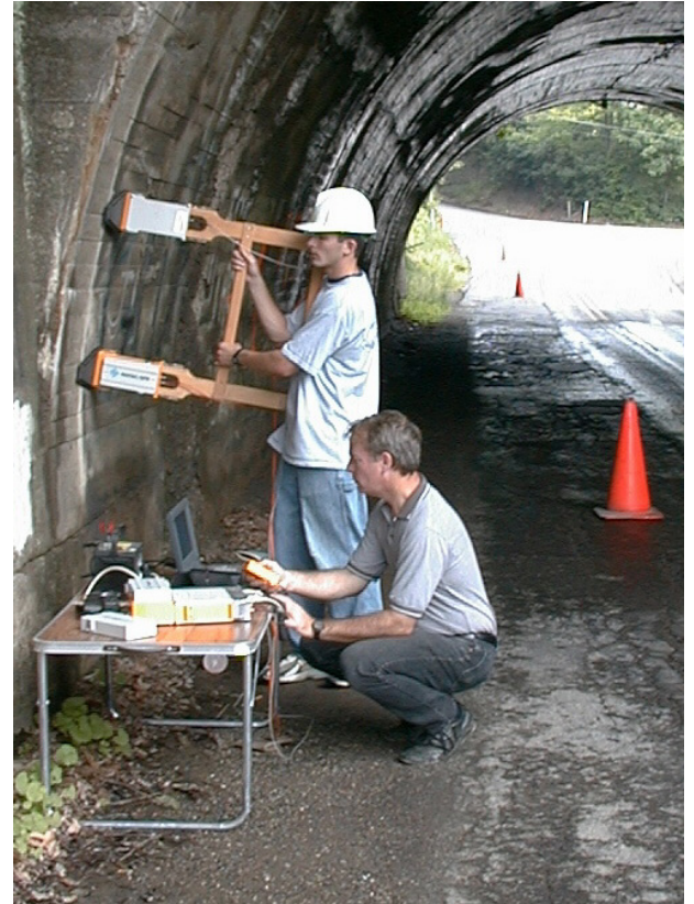
Non-destructive testing of concrete with Ground Penetrating Radar (GPR) at Rich Hill Road test site.
