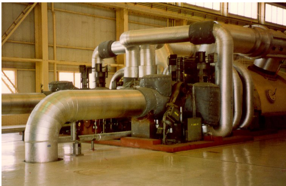
This 110-foot-long by 42-foot-wide turbine pedestal had tilted six inches due to differential movement from underlying expansive clay soil.
