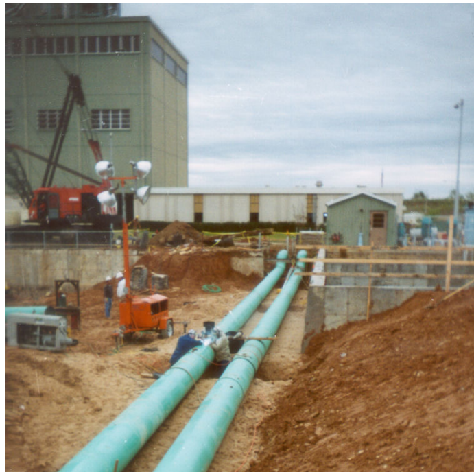
Shallow utility realignment following reconstruction of the cooling water intake canal to address structural distress and Asian clam infestation.
