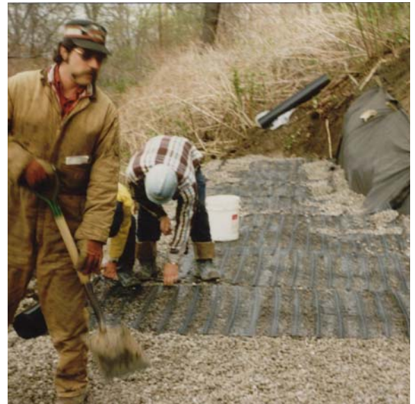
Placement of geogrids during reconstruction of the reservoir slope and bench for railroad track.
