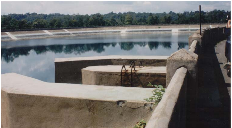
The City of Pittsburgh 114-million-gallon capacity Highland No. 2 reservoir.
