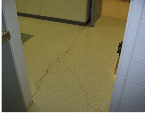
Cracking observed in school building floor.
