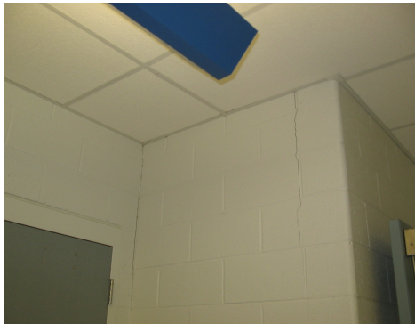
Cracking observed in school building wall.
