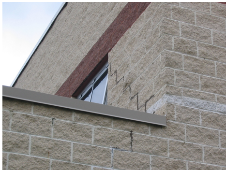
Cracking observed in exterior walls.
