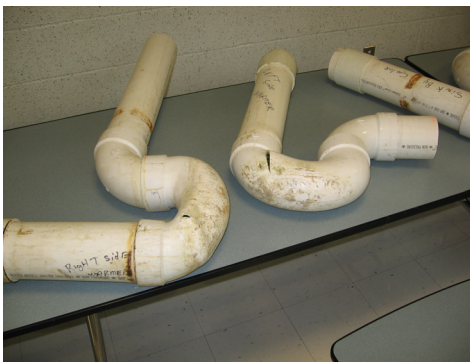
Examples of damaged PVC pipe from building crawl space.
